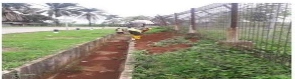
Figure 3. Discovery of a sloping perimeter due to lack of maintenance
